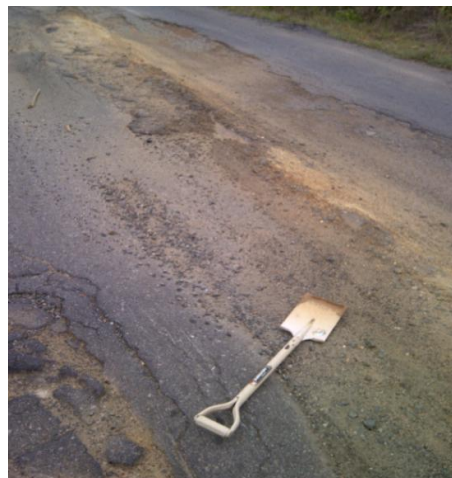
Plate 1. Condition of the road at locality 4 (along Emure-Ekiti/Akungba-Akoko road)
